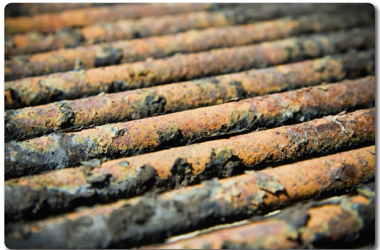
The damaging effects of corrosion
