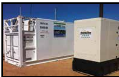
Back-up Power, Australia
