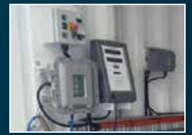
AUTOMATIC TANK GAUGING
