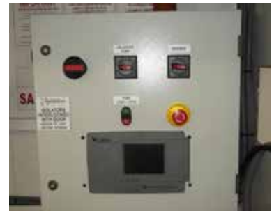
AUTOMATIC TANK GAUGING
