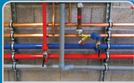
PLUMBING & FIRE SERVICES
