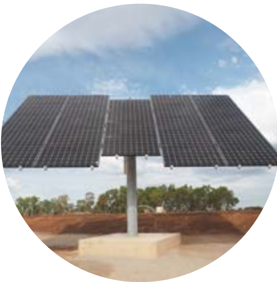
Solar panels at Leonora Wastewater Recycling Facility.
